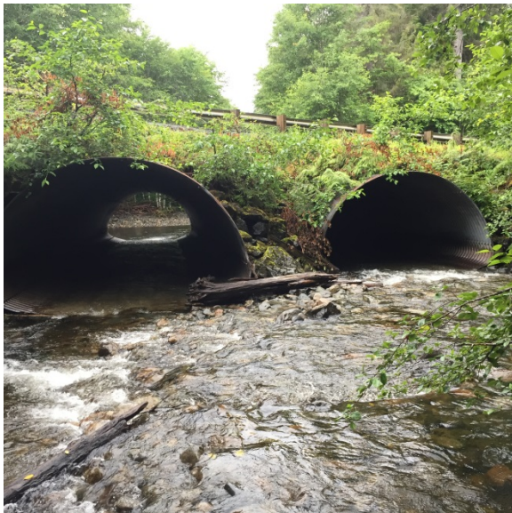
Photo 29. Inlet of double culverts on Threemile Creek crossing the Klawock-Hollis Highway, in the Klawock Lake Watershed, Klawock, Alaska.
