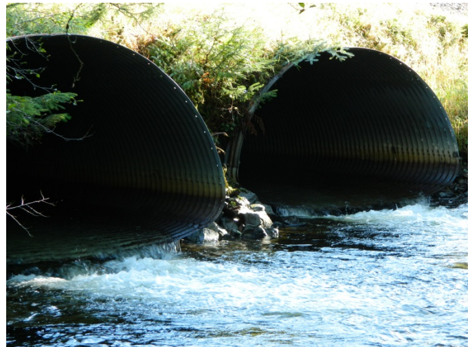
Photo 30. Outlet of double culverts on Threemile Creek crossing the Klawock-Hollis Highway, in the Klawock Lake Watershed, Klawock, Alaska.
