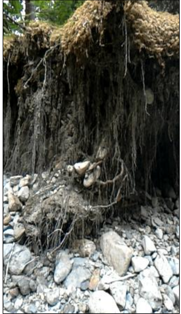
Photo 26: Example of undercut bank and erosion seen throughout the surveyed reaches of Threemile Creek in the Klawock Lake Watershed, Klawock, Alaska.
